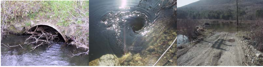
Figure 2: Culvert blocked with woody debris, whirlpool caused by overflow, flooded roadway on the main stem of the Castleton River, reach T02.12.
