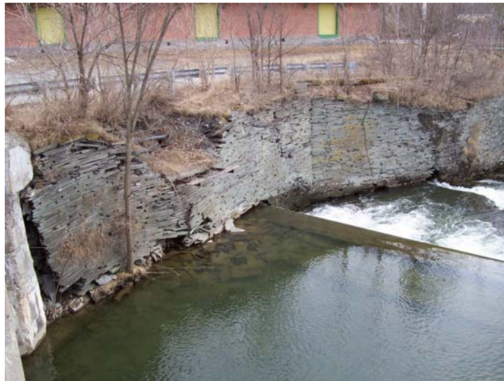
Figure 3: Bank armoring along the main stem of the Castleton River, reach T02.03
